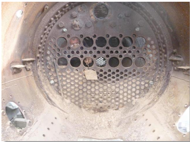
If you look closely you can just see Dave on the other side of the boiler tube plate, shovelling out a mountain of scale.
