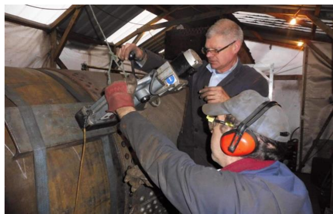
The ‘Chudley Brothers’ in action with the mag drill on the boiler.
