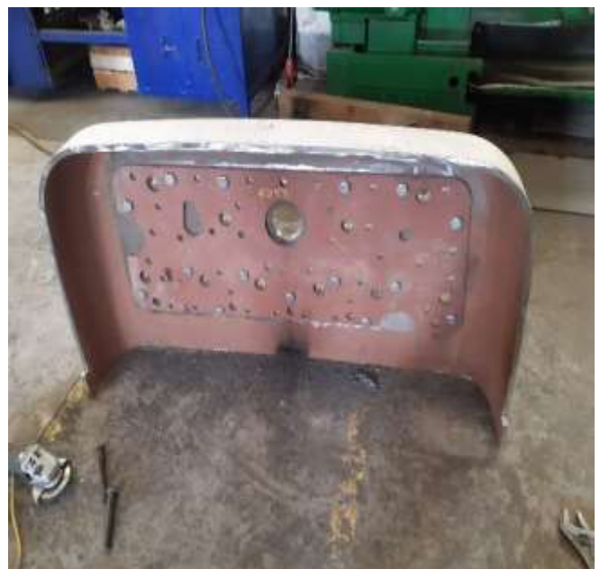
This is the upper section of the boiler back head with the doubling plate, temporarily bolted together for trial fitting.
