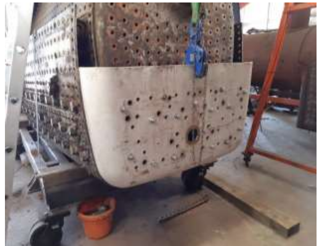
Bearing in mind the boiler is upside down, this is the top section of the back head being trial fitted to the boiler. It certainly looks a good fit from here.
